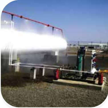
LPG Installation for Industry
