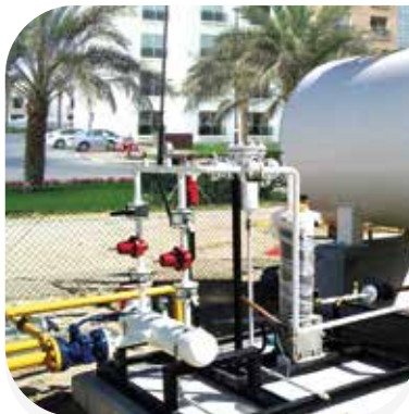
LPG Centralized Gas Distribution for Township
