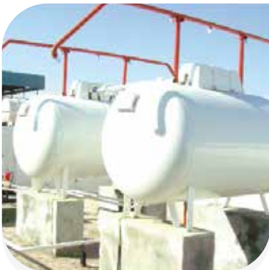
LPG Bulk Installation
