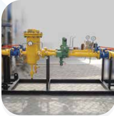
NG Pressure Reducing Station
